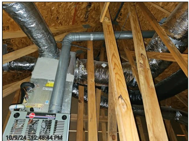
Vent Pipes From Furnace
