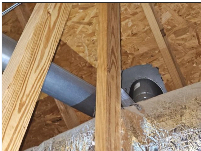
Vent Pipes From Furnace
