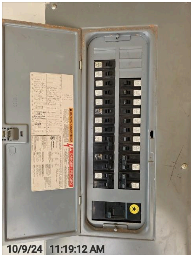
Main Service Disconnect Breaker and Labeled Panel Front
