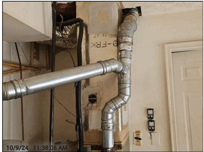
Vent Pipes From Furnace and Water Heater
