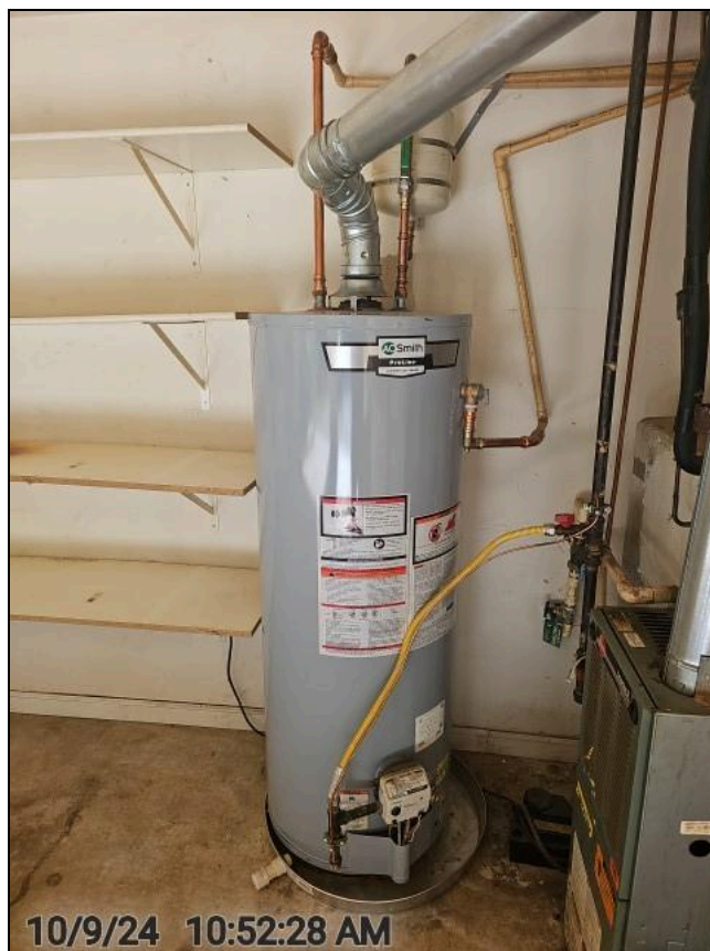
Water Heater and Thermal Expansion Tank
