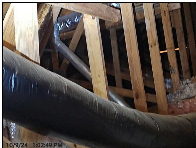
Vent Pipes From Furnace and Water Heater
