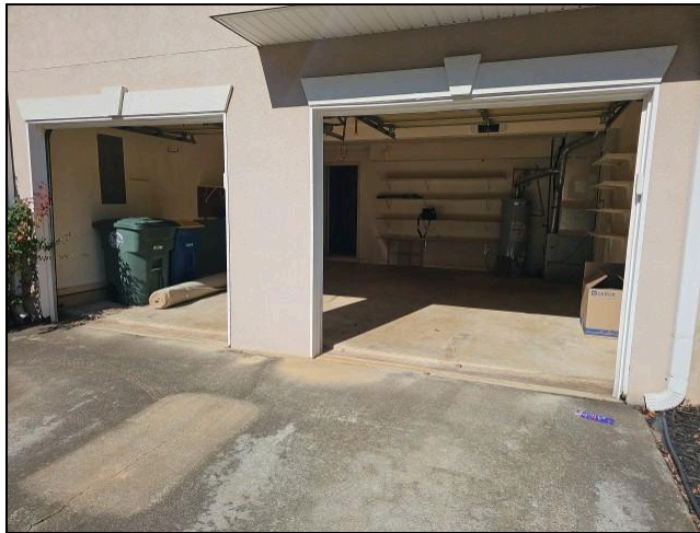
Garage Door and Operator Operational
