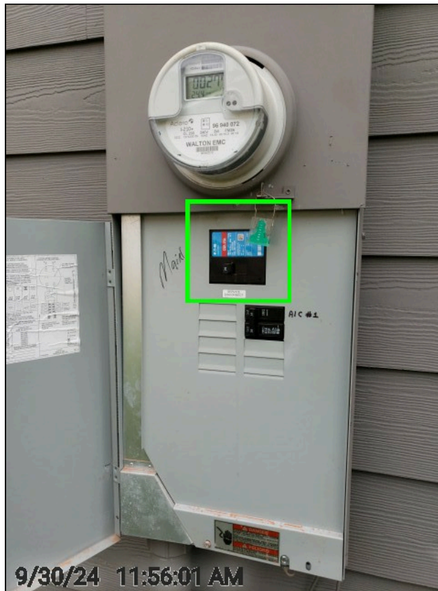
Main Service Disconnect Breaker
