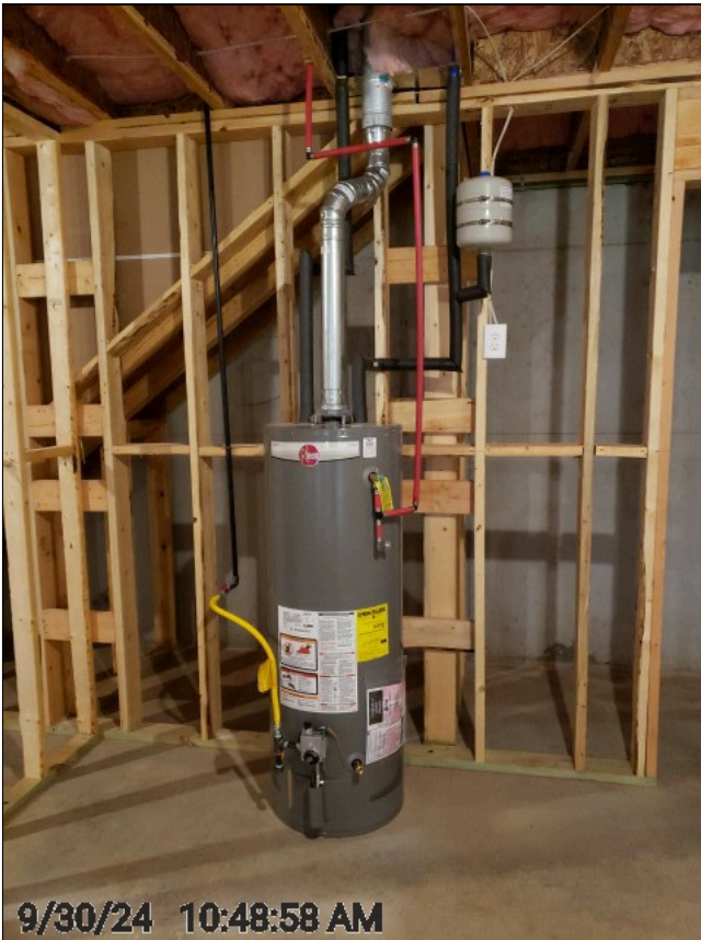
Water Heater and Thermal Expansion Tank
