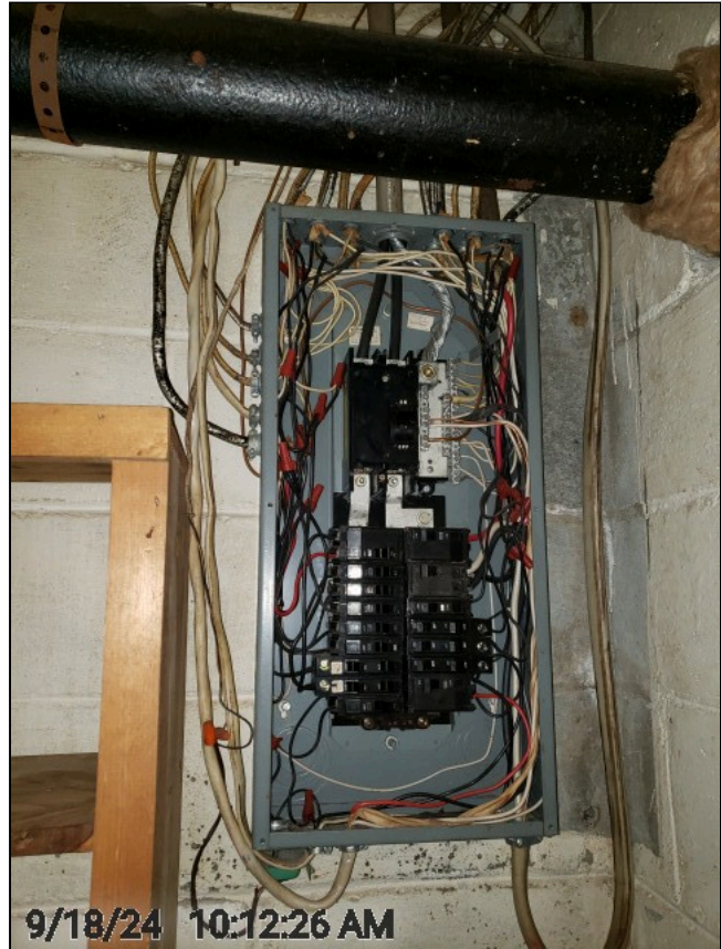
Main Distribution Panel
