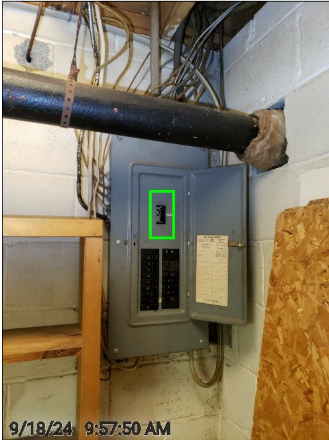
Main Service Disconnect Breaker
