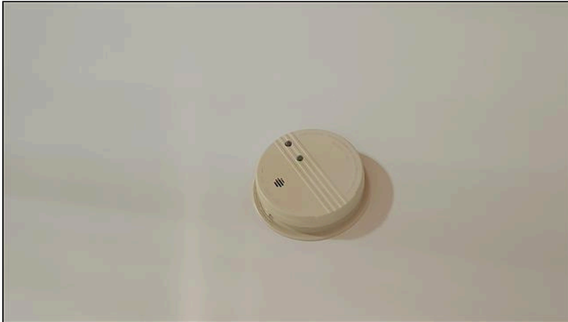
Smoke detector upstairs hall
