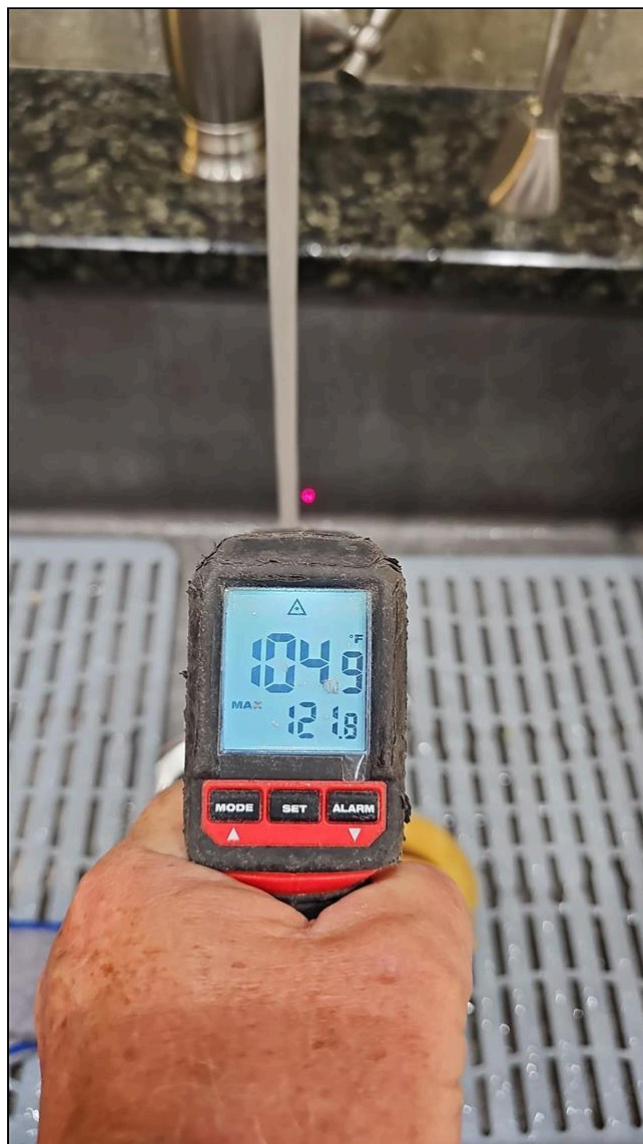
Water Heater Delivering Heated Water
