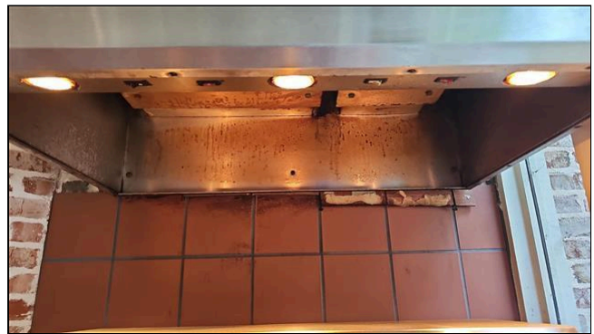
Exhaust Vent Above Grill
