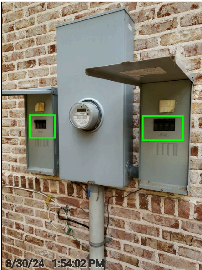
Main Service Disconnect Breakers
