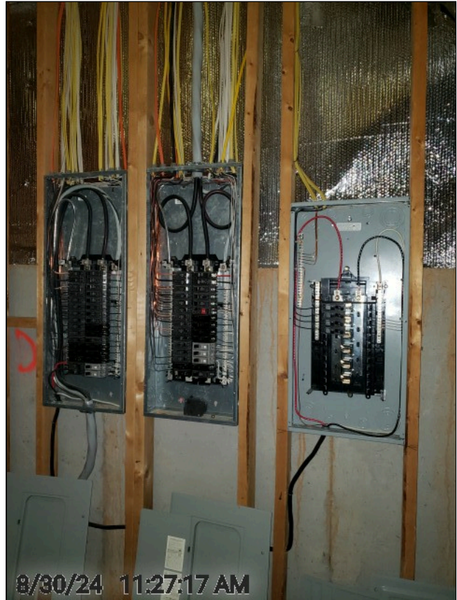
8/30/24 11:27:17 AM Distribution Panels
