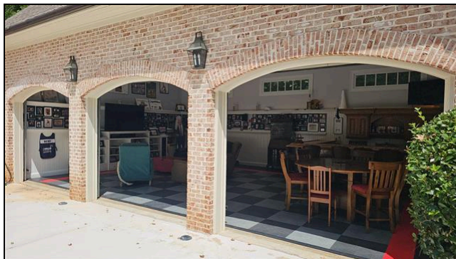
Garage Door and Operator Operational
