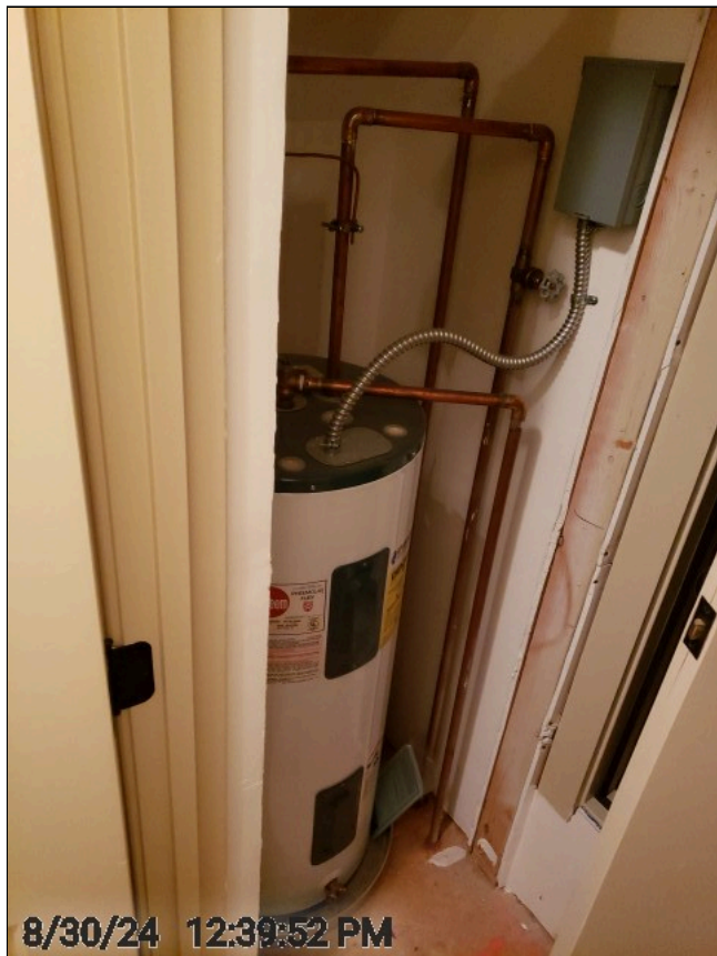
Water Heater Bonus Room
