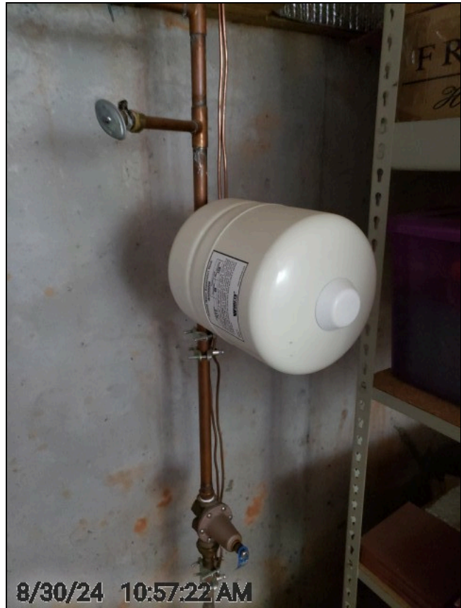
Thermal Expansion Tank
