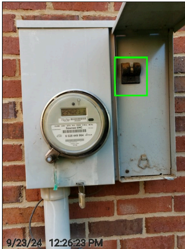
Main Service Disconnect Breaker
