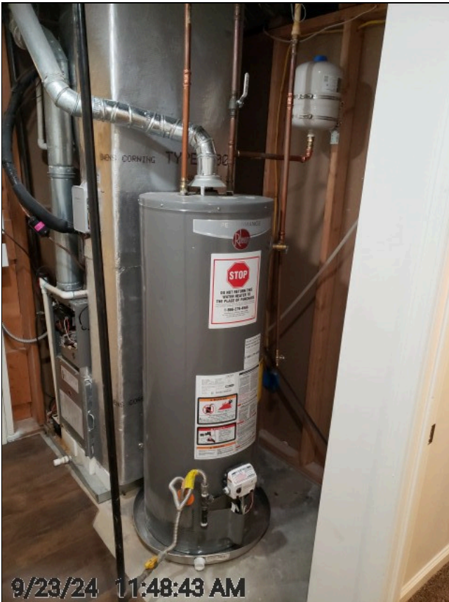
Water Heater and Thermal Expansion Tank
