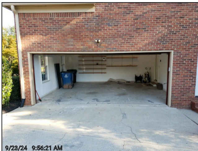
Garage Door and Operator Operational
