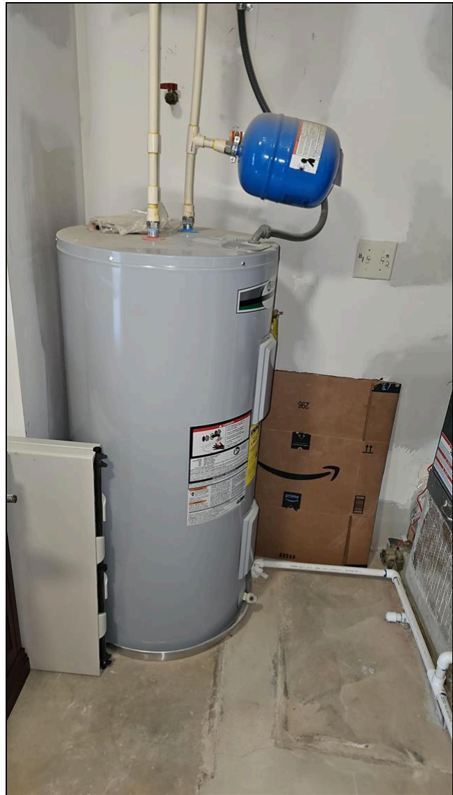
Water Heater and Thermal Expansion Tank
