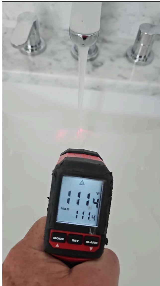
Tankless Water Heater Delivering Heated Water
