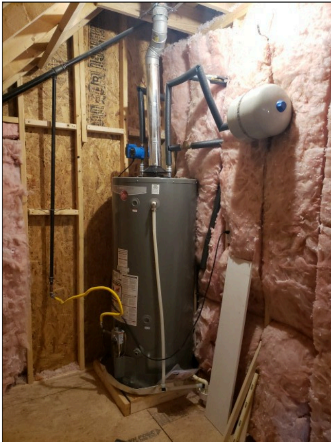
Water Heater and Thermal Expansion Tank
