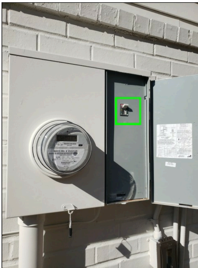
Main Service Disconnect Breaker
