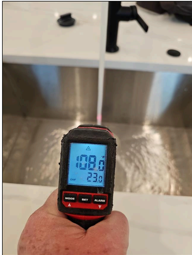
Water Heater Delivering Heated Water
