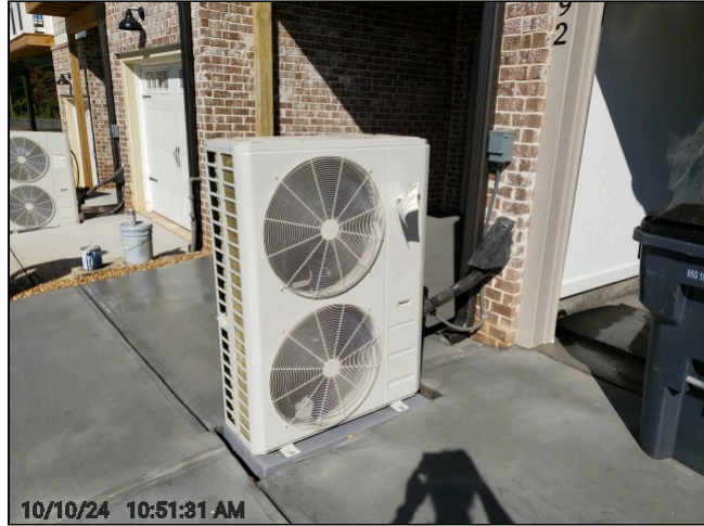
Heat Pump Condensing Unit
