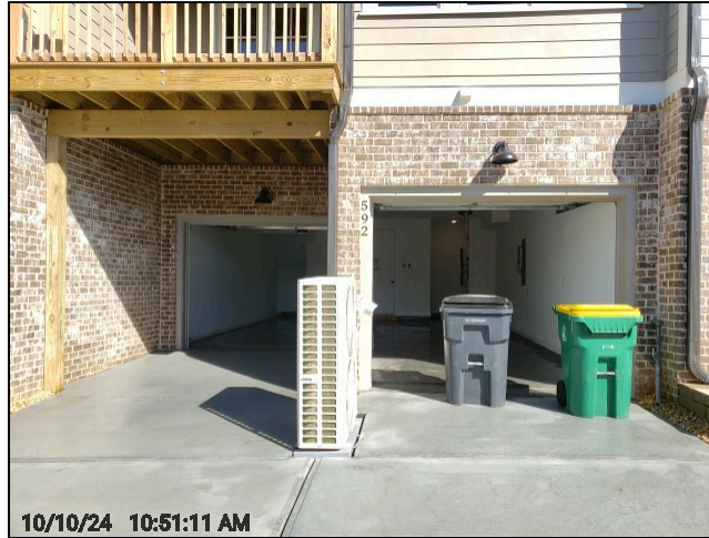
Garage Door and Operator Operational
