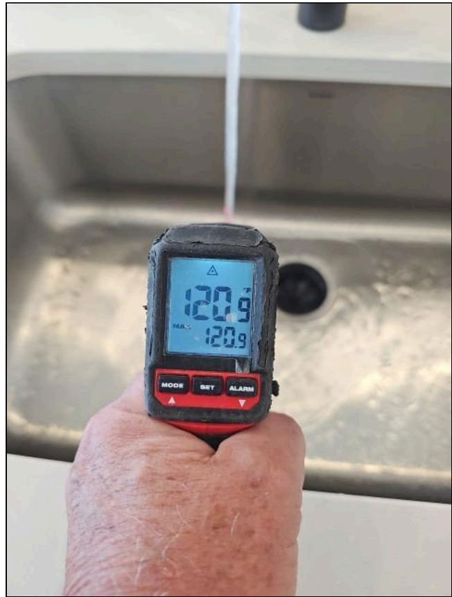
Water Heater Delivering Heated Water
