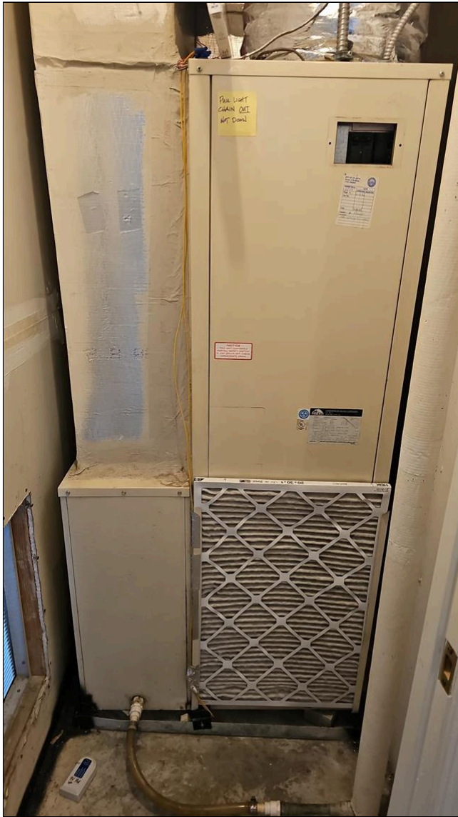
Packaged HVAC System
